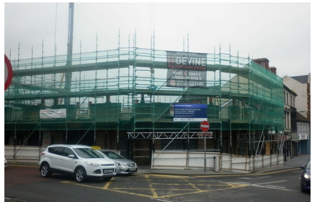
New build social housing under construction at Main Street, Strabane, being delivered by Ark Housing Association.
