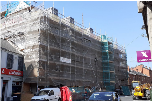
New build social housing under construction at Patrick Street, Derry/Londonderry, being delivered by Triangle Housing Association.
