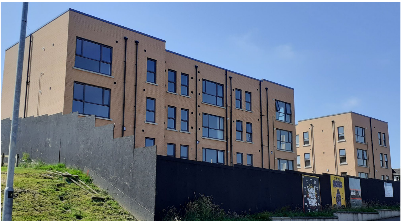
New build social housing under construction at Mimosa Court, Derry/Londonderry, being delivered by South Ulster Housing Association.
