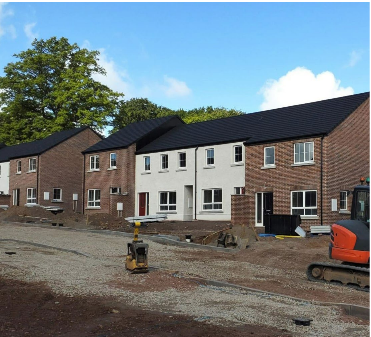
This photo shows the new build scheme at Old English Road, Dungannon (Choice HA) which is currently on site.
