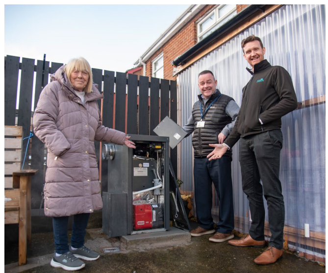
This photo shows a tenant from Dungannon with her newly installed boiler
