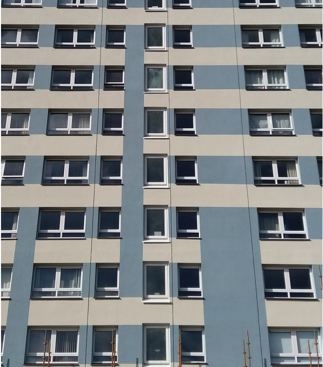
StoTherm Vario External Wall Insulation (EWI) at Garnet House
