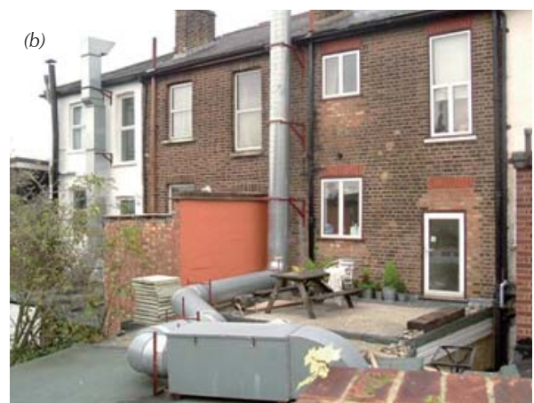
Figure 14: Examples of Category 1 hazards for falls between levels
