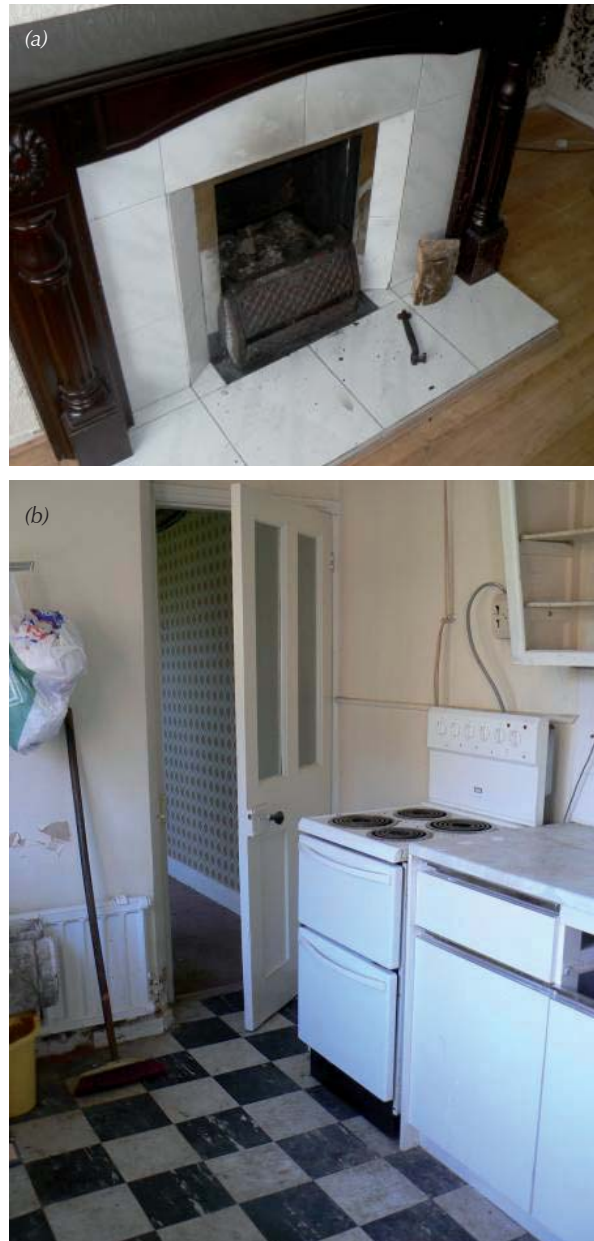
Figure 22: Examples of Category 1 hazards for fire and hot surfaces and materials
