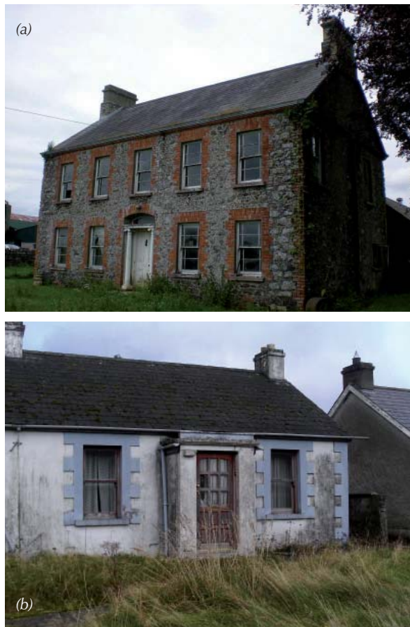
Figure 16: Examples of Category 1 hazards for excess cold (a) Pre-1919 detached dwellings make up 37% of NIHCS 2009 dwellings with Category 1 excess cold hazards – this dwelling has solid fuel fires, no insulation and draughty sash windows, and has a SAP rating of 1 (b) A rural bungalow with a SAP rating of 16
